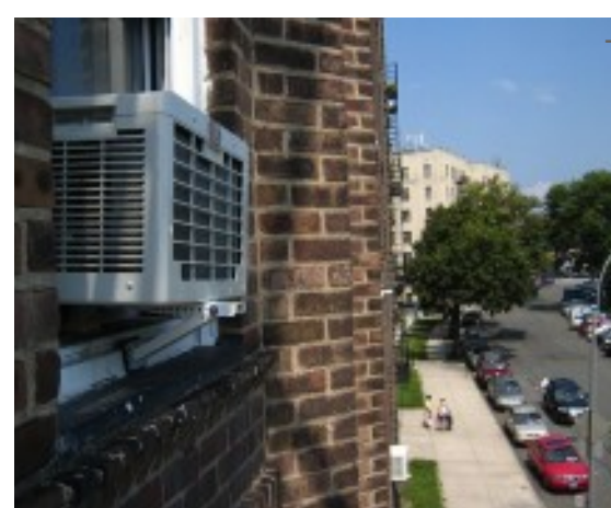
Shade Your Air Conditioner to Save Money on Electricity
